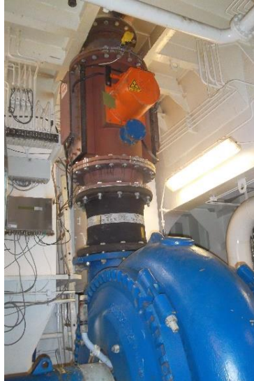
Figure 8. The RF density measurement prototype as installed inside the pump room of the CORNELIS SENIOR. The signal conditioner (silver box, to the left) is also visible
